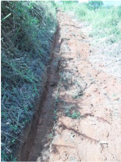
Soft sections of pipeline
